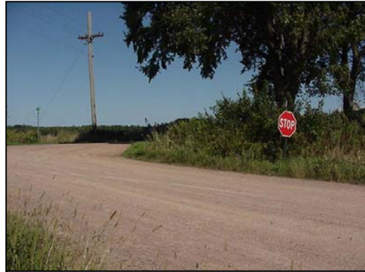
Local road intersection visibility should be maintained.
