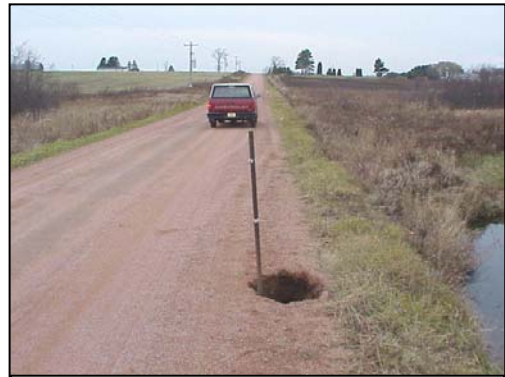
Local road maintenance issues, rural Clark County
